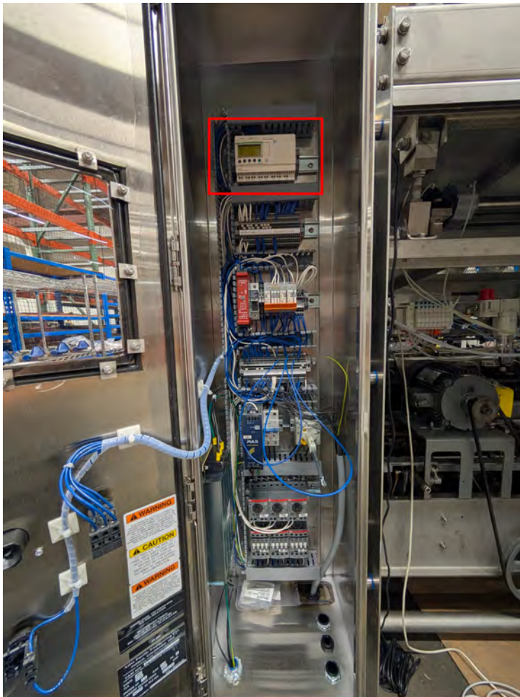
Control panel located in PRO electrical box.
