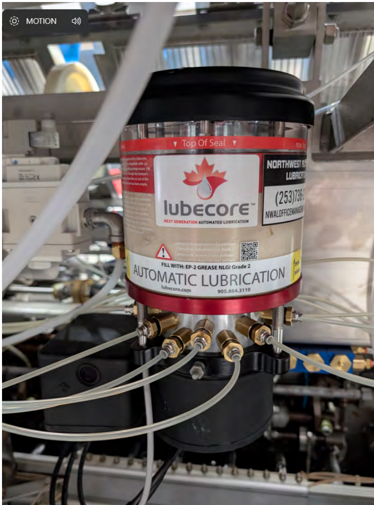
Picture of Auto Lube System.
